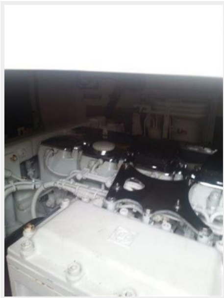
Engine & Mechanical Equipment 2
