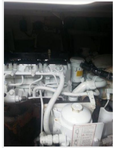
Engine & Mechanical Equipment 1
