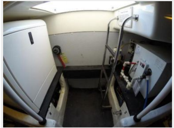
Engine Room (facing Aft)
