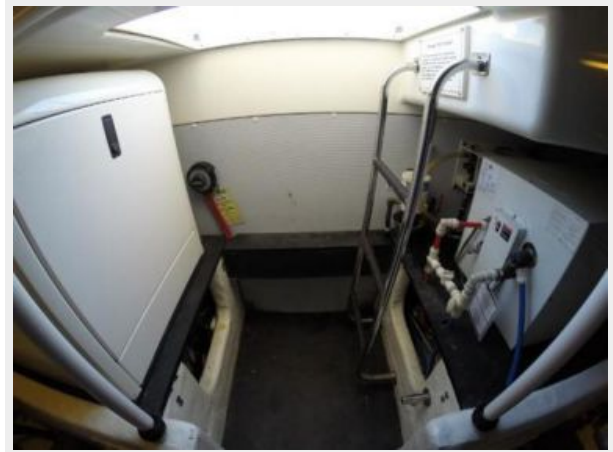
Engine Room (facing Aft)
