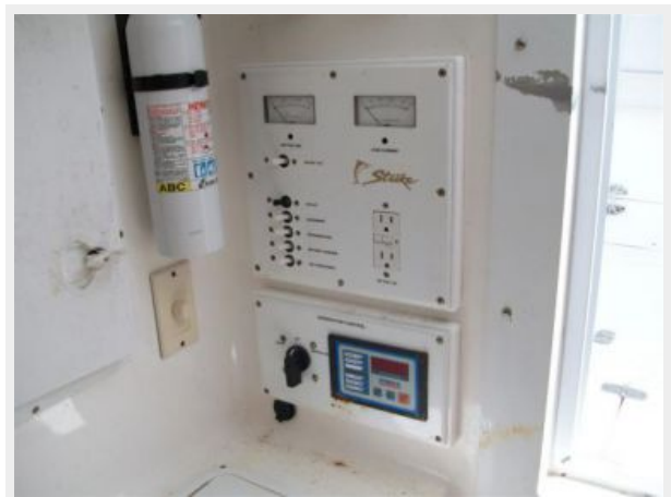
Electric panel - ready for generator hook up
