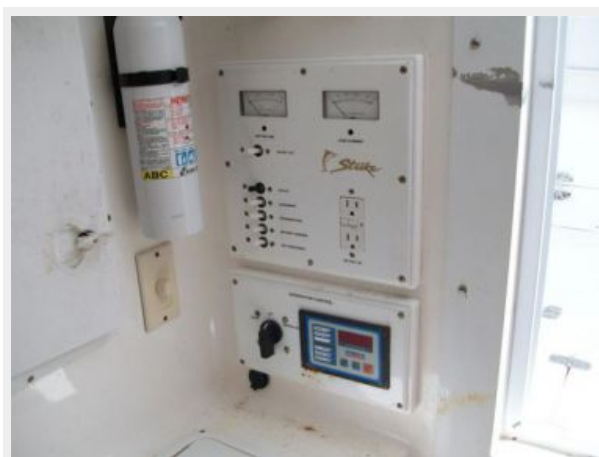
Electric panel - ready for generator hook up
