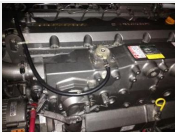
Spotless engine room
