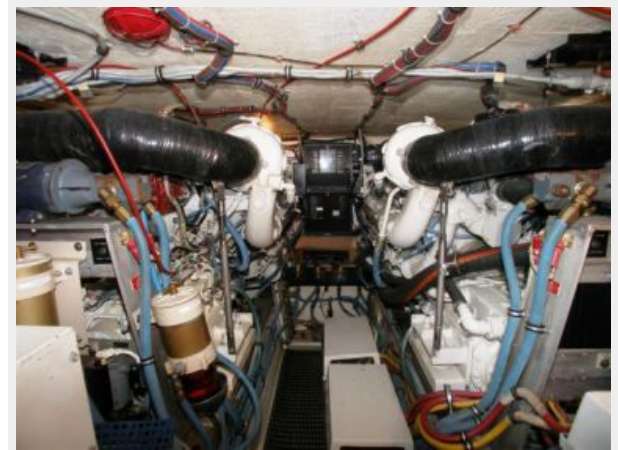
Engine Room View Forward
