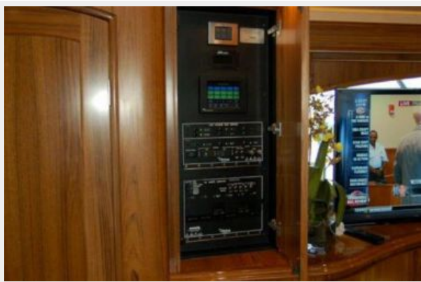
Electrical Panel in Salon
