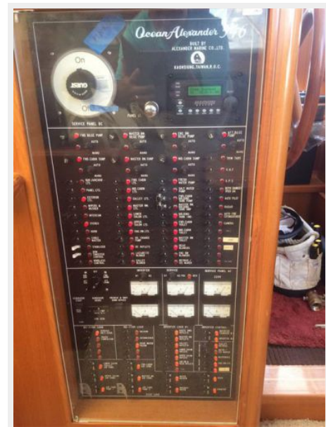
Main electric panel
