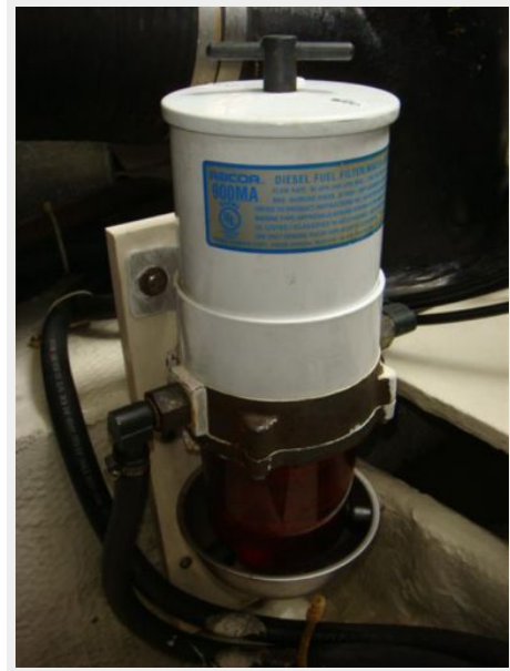
38' Regal port main engine Racor fuel filter
