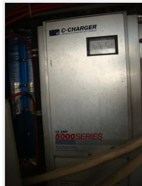
38' Regal battery charger
