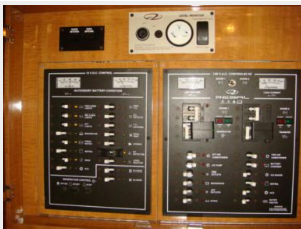
38' Regal electrical panel
