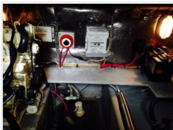
Engine room forward
