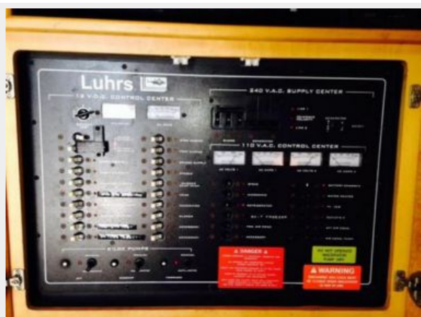
Ships electrical panel
