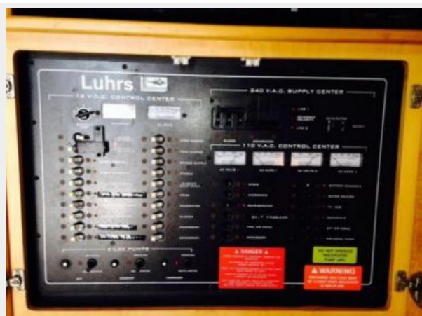
Ships electrical panel
