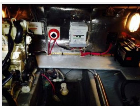
Engine room forward
