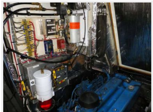
Engine Room, View of Engine
