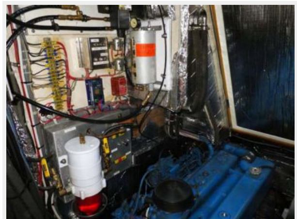
Engine Room, View of Engine
