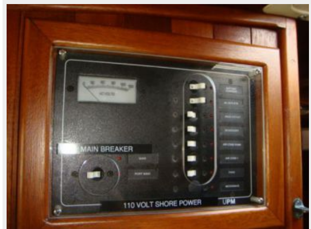
26' Pemaquid Beach electrical panel
