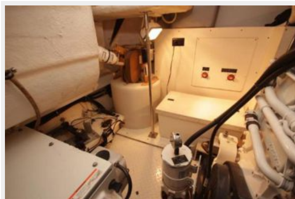
Engine Room Starboard Aft
