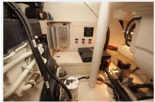
Engine Room Port Aft
