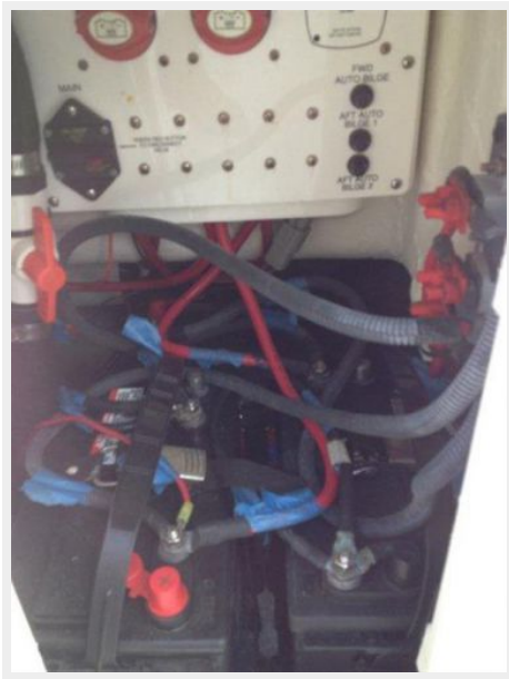
Electrical System / Equipment - Batteries
