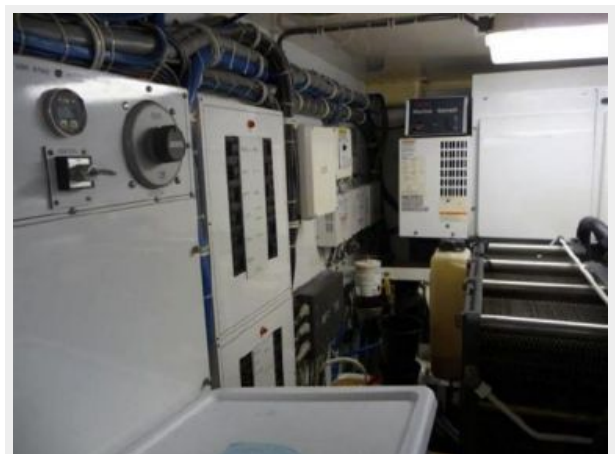
Engine Room Forward
