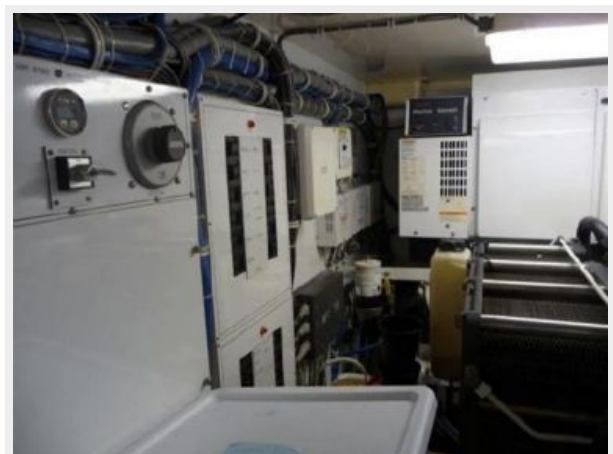
Engine Room Forward
