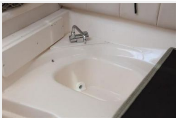
Wash down sink
