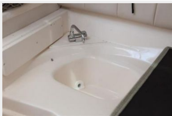
Wash down sink
