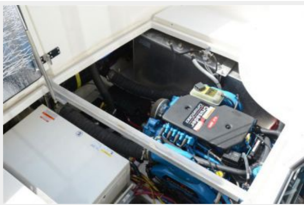
Starboard Motor & Generator
