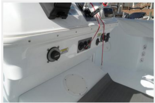
2004 34' Baja Sportfish Battery Switches
