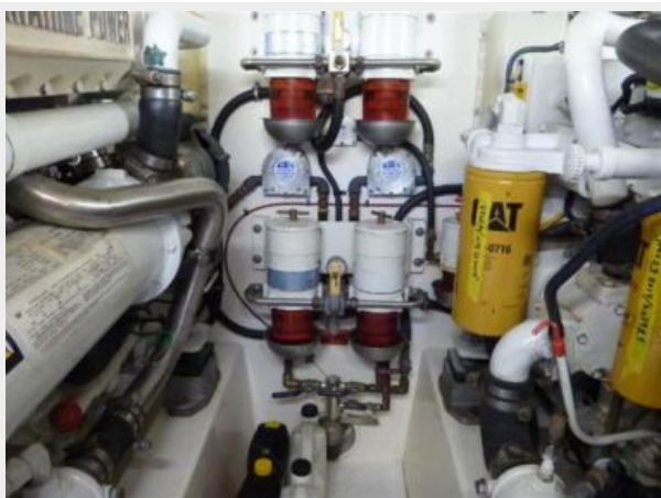
Clean Engine Room
