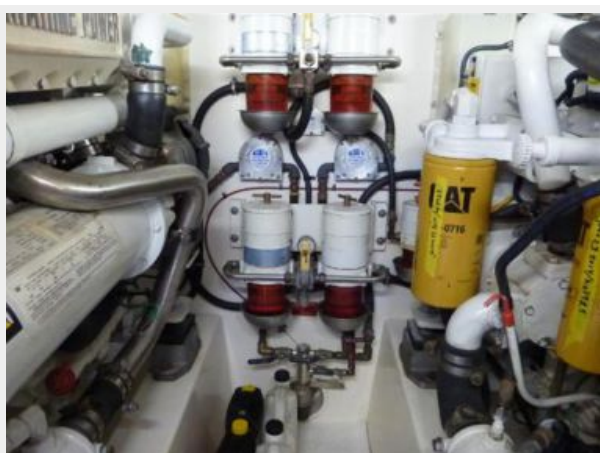
Clean Engine Room
