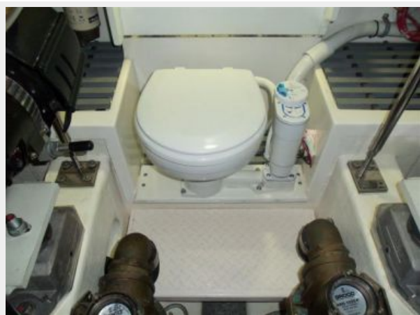
Custom Engine Room Toilet
