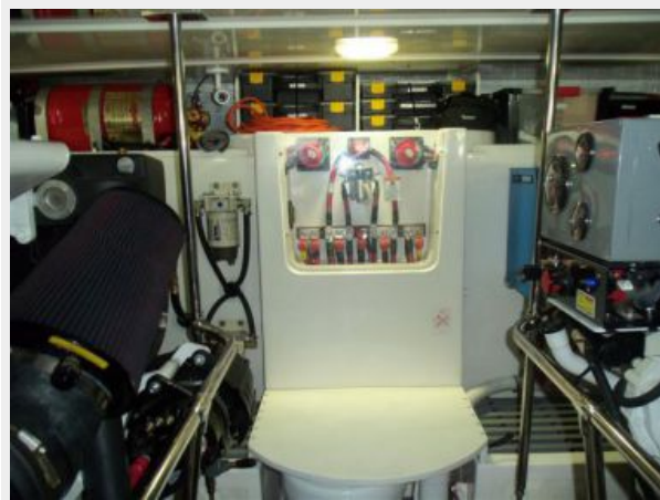
Engine Room Forward
