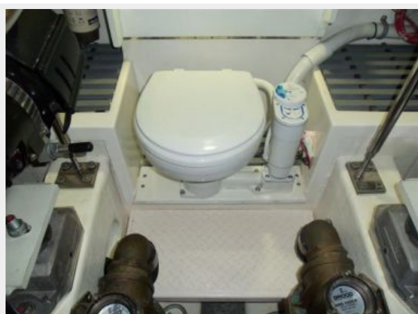
Custom Engine Room Toilet
