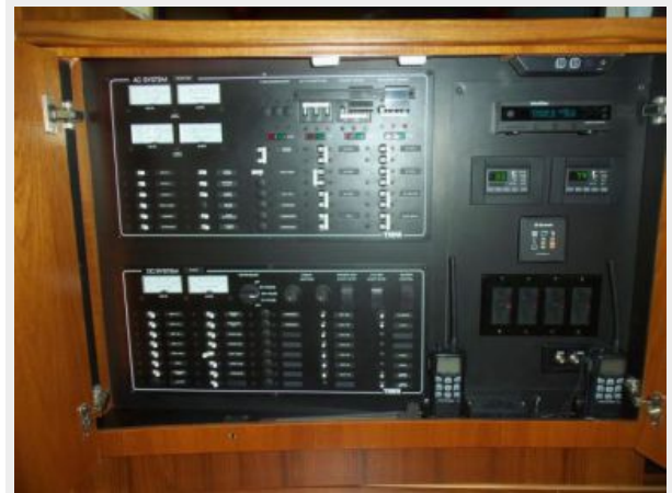
Salon Electrical Locker
