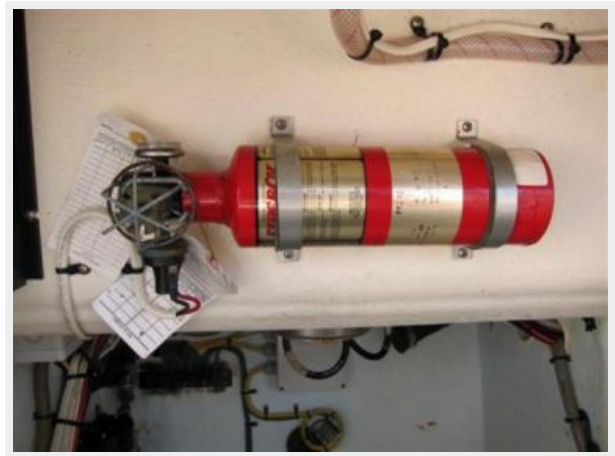
Fire suppresant system
