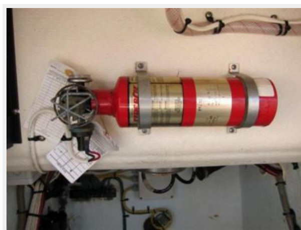
Fire suppresant system
