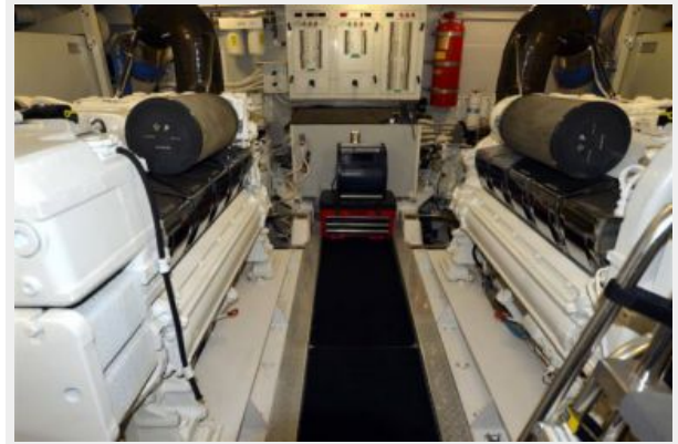
Engine room looking forward
