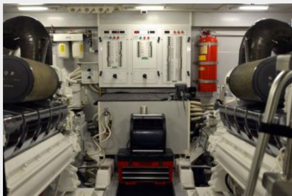
Engine room looking forward (3)
