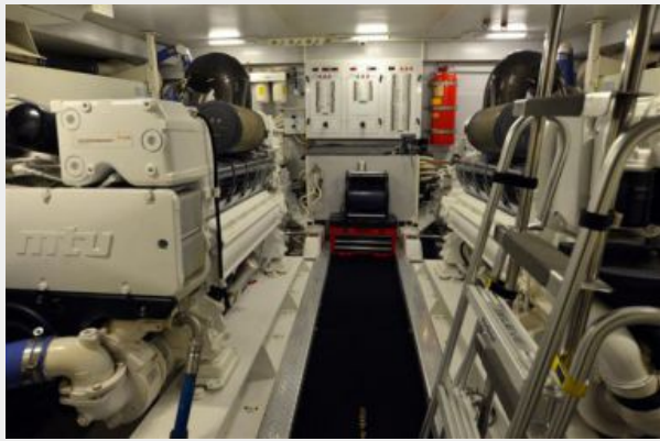
Engine room facing forward
