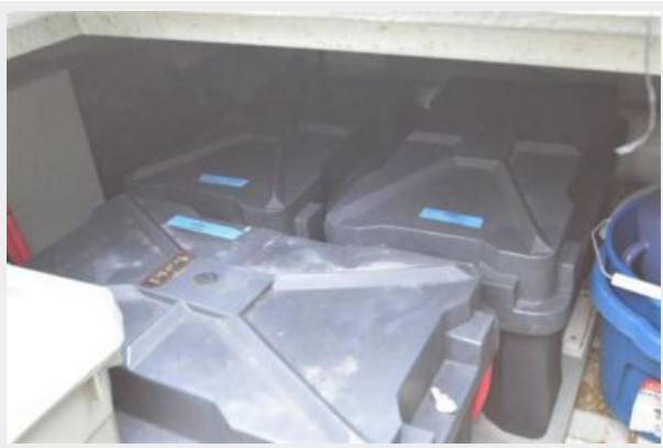
Lazarette New Batteries
