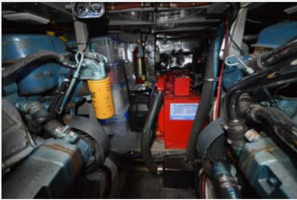
Engine Room Forward
