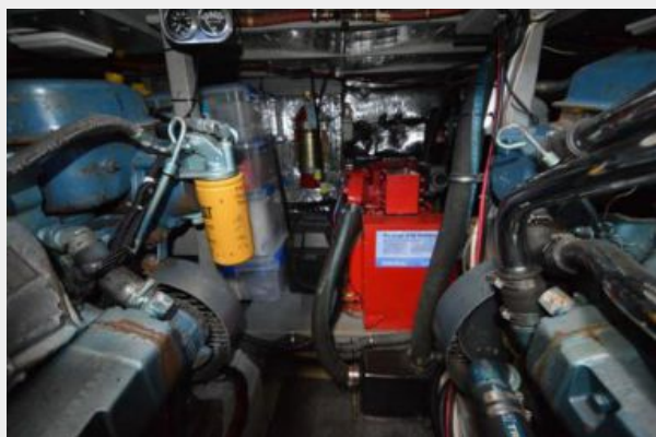
Engine Room Forward
