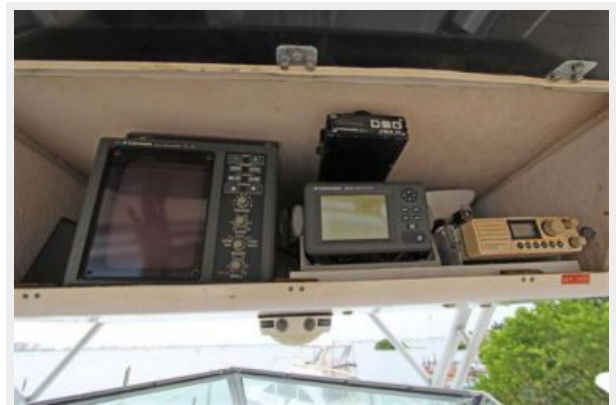
Overhead Electronics Box
