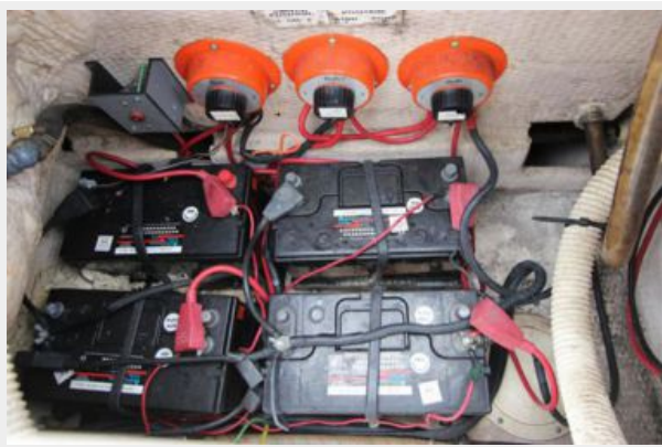
4-Marine Battery's & Switches
