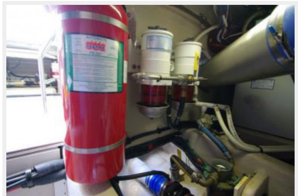
Fire Extinguishing System
