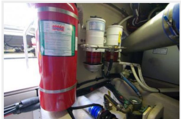
Fire Extinguishing System
