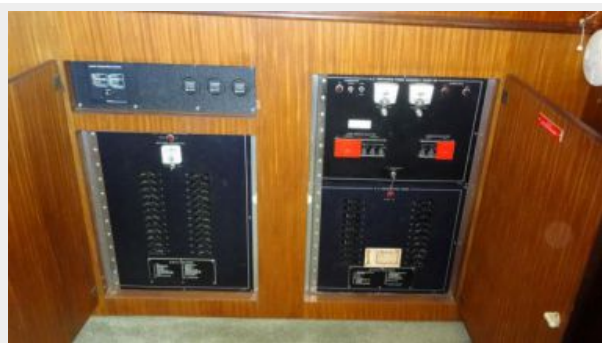
AC / DC Breaker Panels
