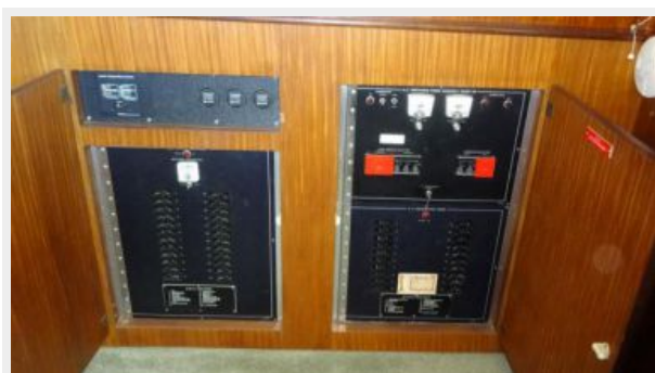
AC / DC Breaker Panels
