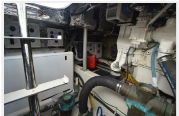
Engine Room and Generator
