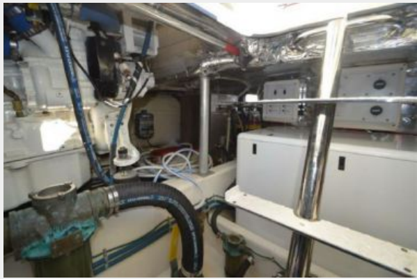
Engine Room and Generator
