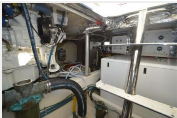
Engine Room and Generator
