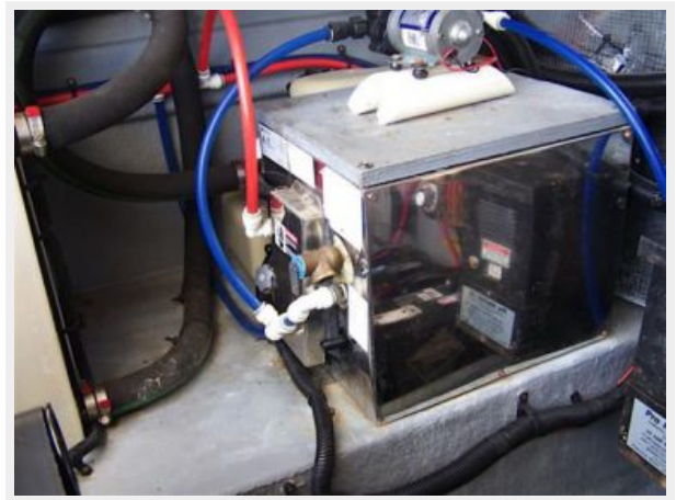
Hot Water Heater
