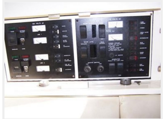
Main Distribution Panel
