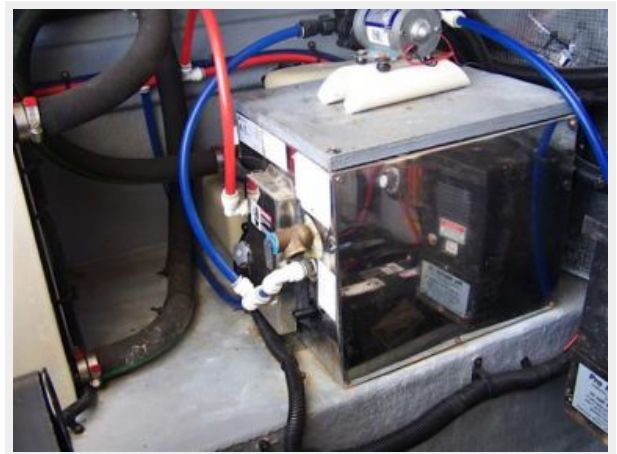
Hot Water Heater
