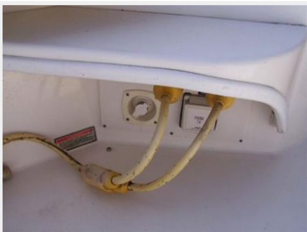
Shore Power Connection
