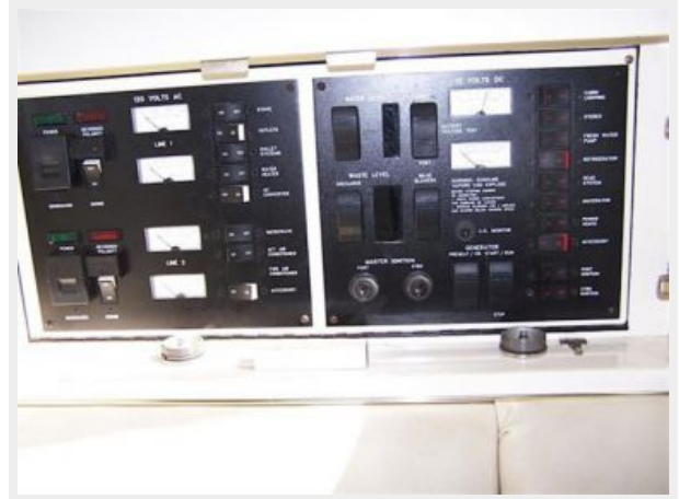
Main Distribution Panel
