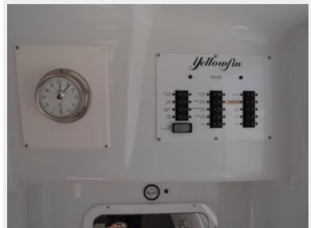
Electrical Panel & Clock
