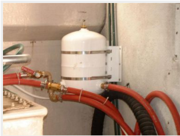
Part of new hydronic hot water heating system for cold weather operation up North!
