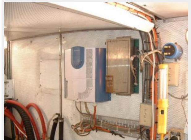
Recent Mastervolt 24V charger...also Kohler 15K (?) newer genset
