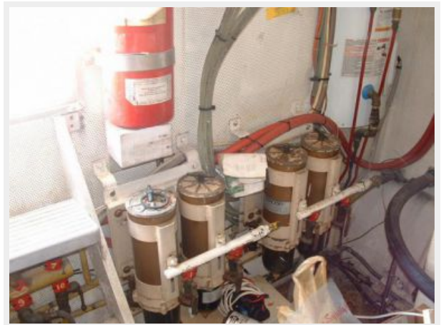
All filters and valves are easy to maintain and not many tight spaces!
