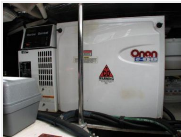
Electrical System / Equipment - Genset
