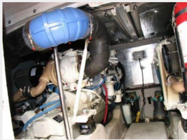
Engine & Mechanical Equipment 1 - Port Engine
