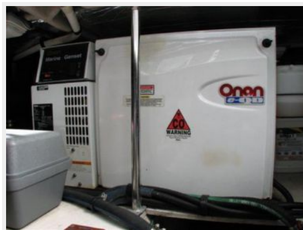
Electrical System / Equipment - Genset
