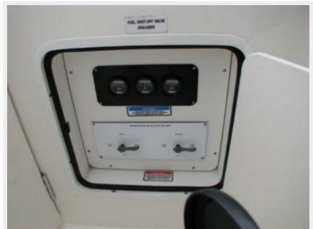
Engine & Mechanical Equipment 4 - Fuel Manifold
