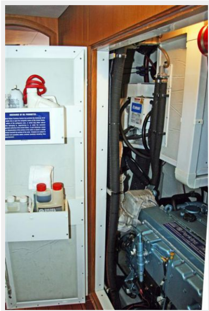
Door to Engine Room
