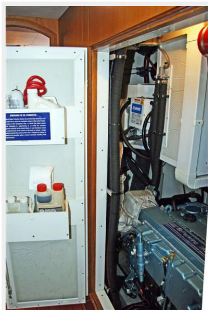
Door to Engine Room
