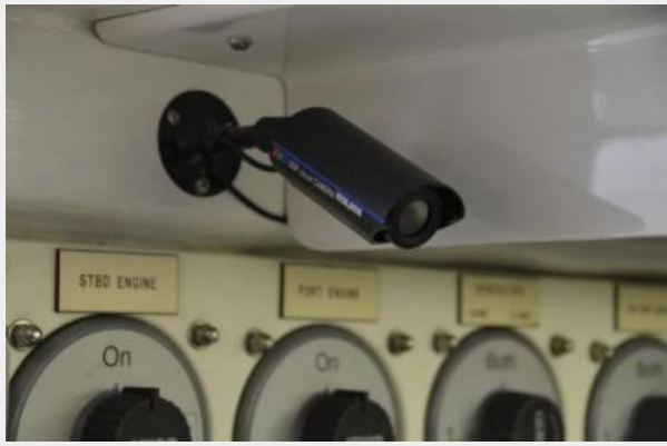
58 Davis Engineroom Camera
