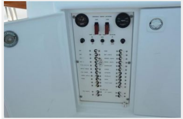
58 Davis Bridge Electrical Panel
