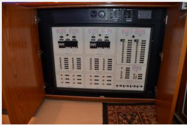
58 Davis Electrical Panel
